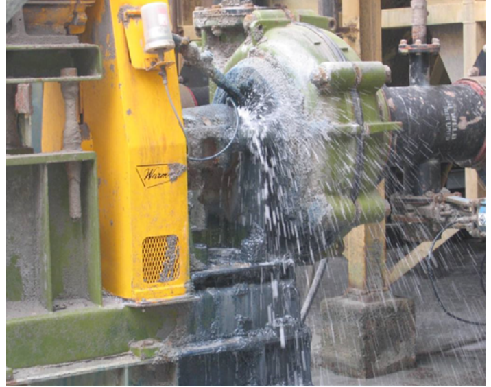
Result of a leaking shaft sleeve
